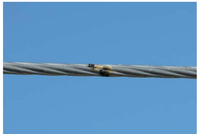
Figure 2 – Burned contact point on 13.8-kV power line
