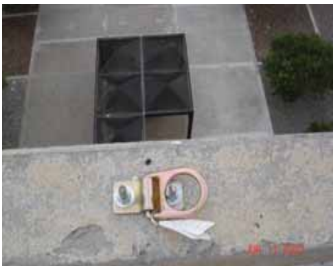
Figure 2-1. Fall protection anchor bolted in position. Note: The canopies are 45 - 50 feet below.
