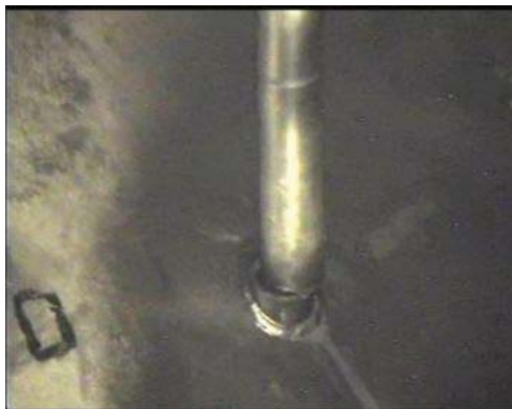
Figure 3-3. Failed pipe nozzle on tank head
