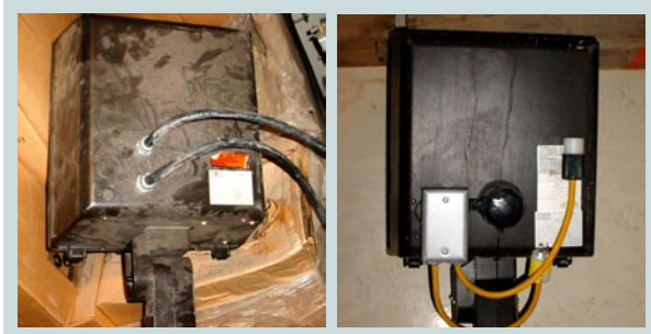
Figure 2-4. Back of previously modified (left) light unit and corrected modification (right)
