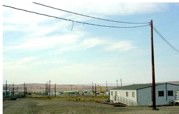
Figure 1-3. Cut power line running diagonally across the road bed
