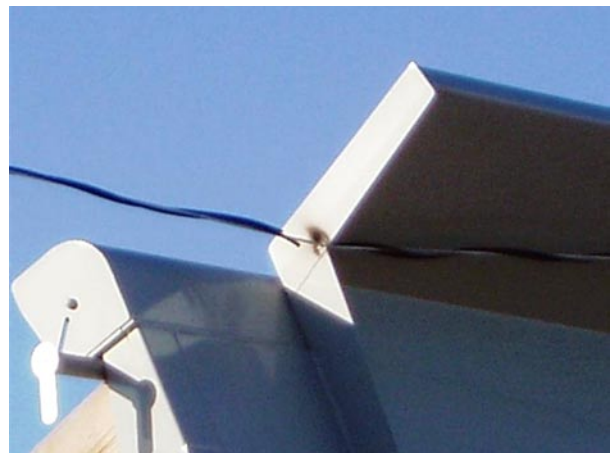
Figure 1-2. Severed power line held in place by support cable
