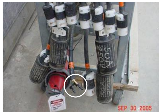
Figure 4-1. Pigtails on the back of the mini load center and the exposed wires that arced (circled)
