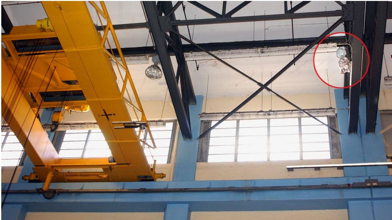
Figure 2-1. Broken light fixture
