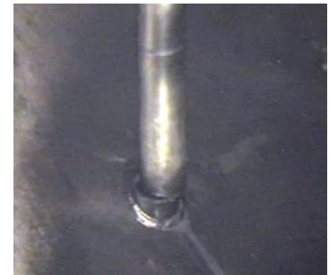
Figure 4-2. Failed pipe nozzle on tank head
