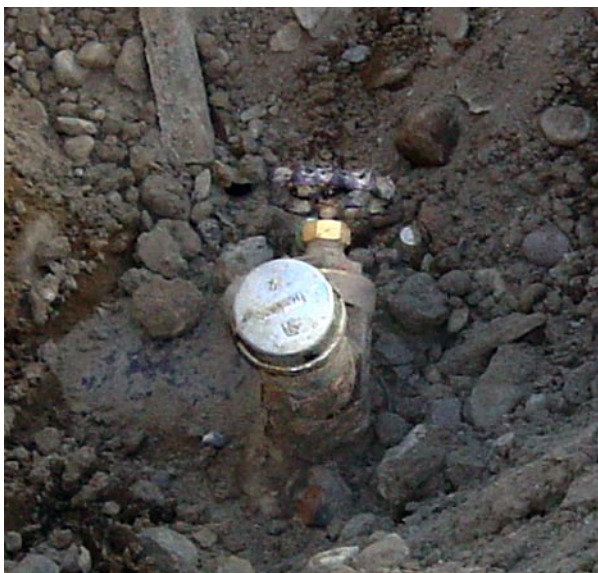
Figure 3-3. Chlorination stub attached to water main
