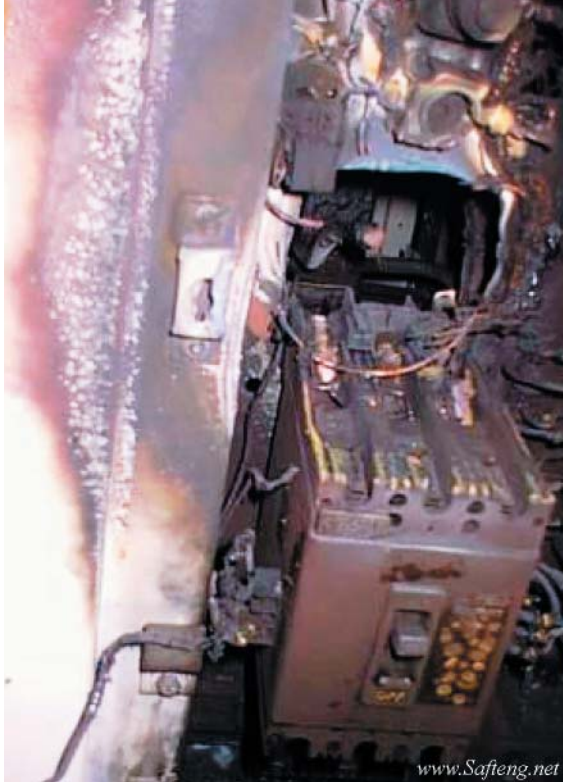
Figure 4-2. Damaged electrical cabinet
