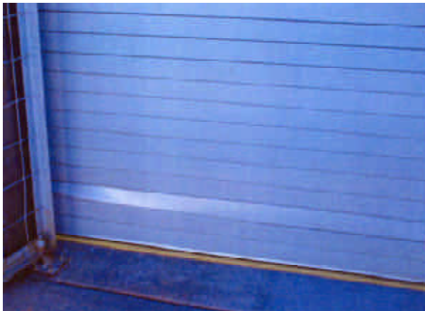
Figure 2-2. Buckled door slat (Rocky Flats)
