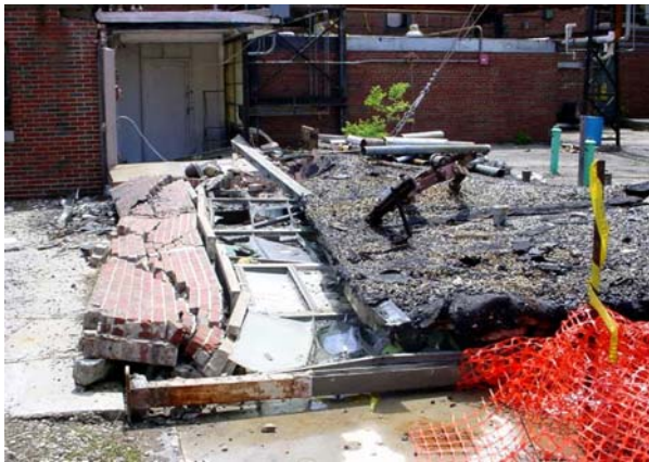
Figure 1-1. The collapsed breezeway
