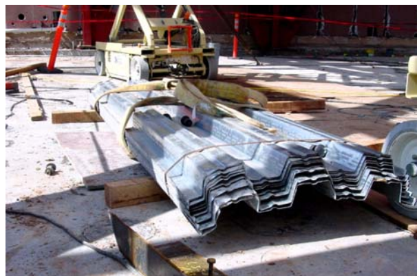
Figure 3-1. Dropped decking material
