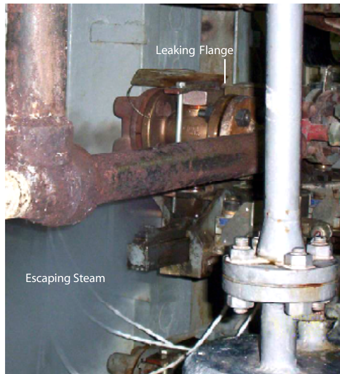
Figure 2-1. Actual steam leak
