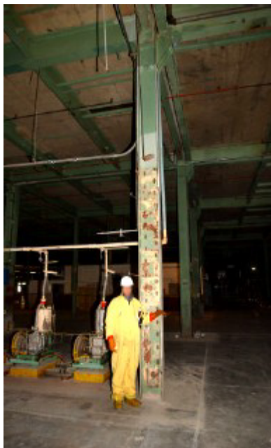
Figure 4-1. Wide-flange column involved in the accident (blocks removed)
