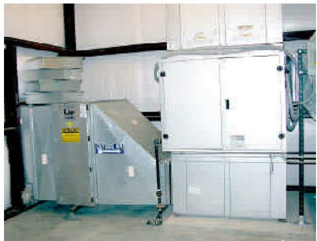
Figure 3-1. Direct-fired furnace (on right)
