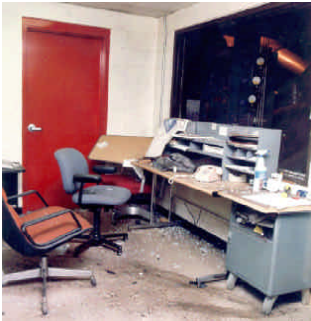
Figure 2-2. The control room window was shattered
