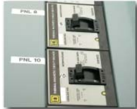
Figure 5-2. 200-amp circuit breakers showing thick tapered actuation handle
