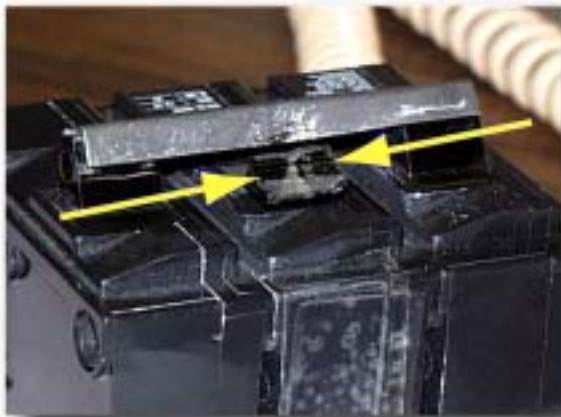
Figure 5-4. Damaged circuit breaker handle
