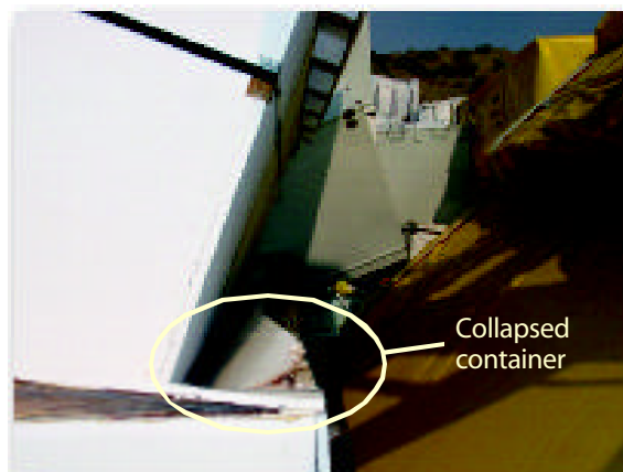
Figure 4-3. Container that collapsed
