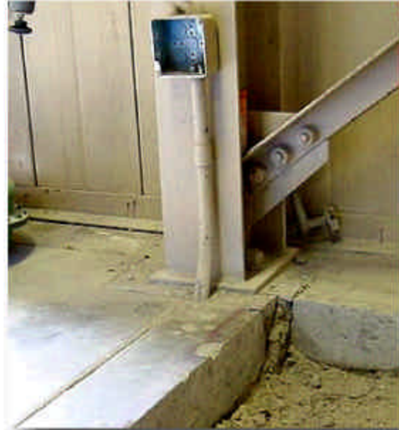
Figure 1-1. Electrical receptacle and conduit penetrating the floor and the location of the saw cut
