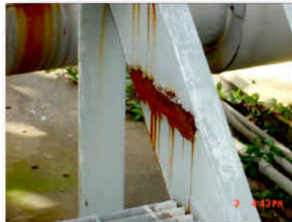
Figure 3-2. Corrosion where stair tread attached to the frame
