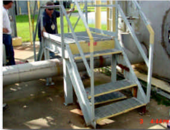
Figure 3-1. Stairs after the incident, with the broken step on the ground
