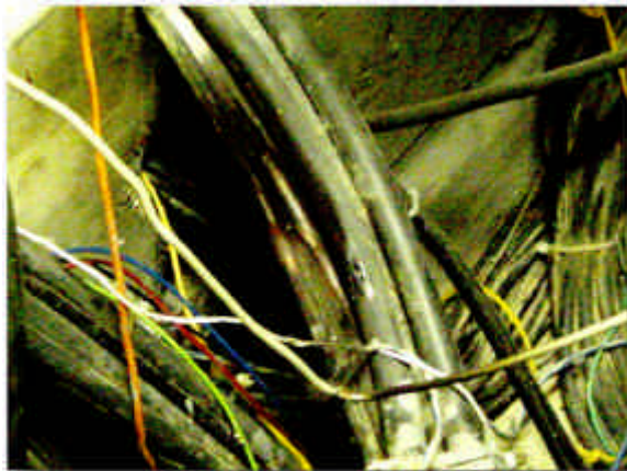
Figure 2-3. Damage to 480-volt cable and small white ground wire
