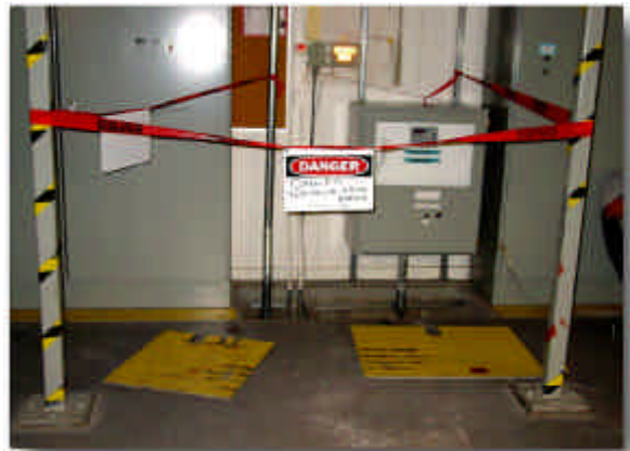
Figure 2-1. Cable trench and cover plates
