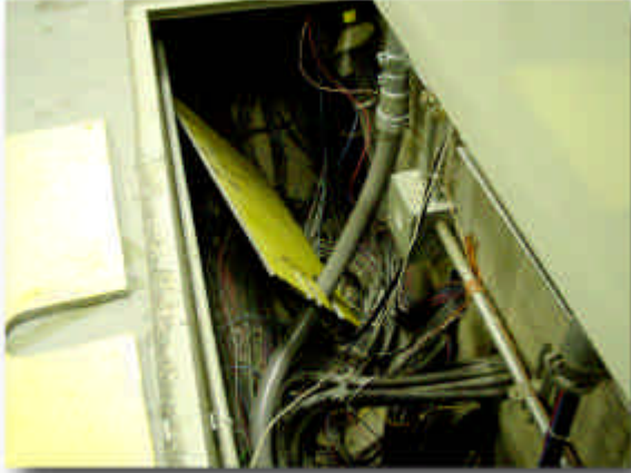
Figure 2-2. Smaller plate in trench following incident
