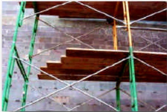
Figure 2-2. Example of scaffolding with deficient spacing
