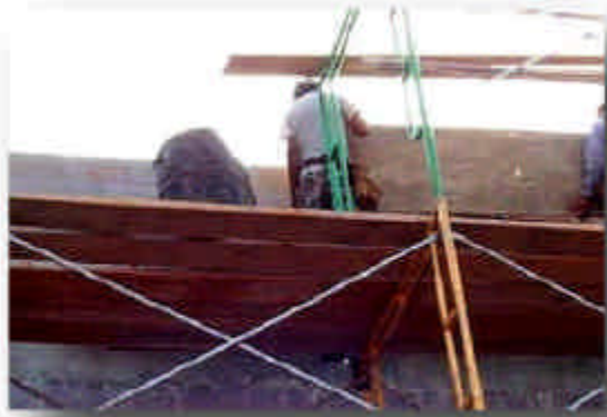
Figure 2-1. Example of scaffolding without handrails or toe boards
