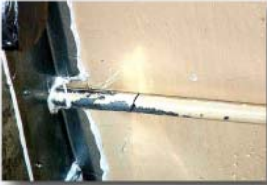
Figure 1-5. Cut electrical conduit during
