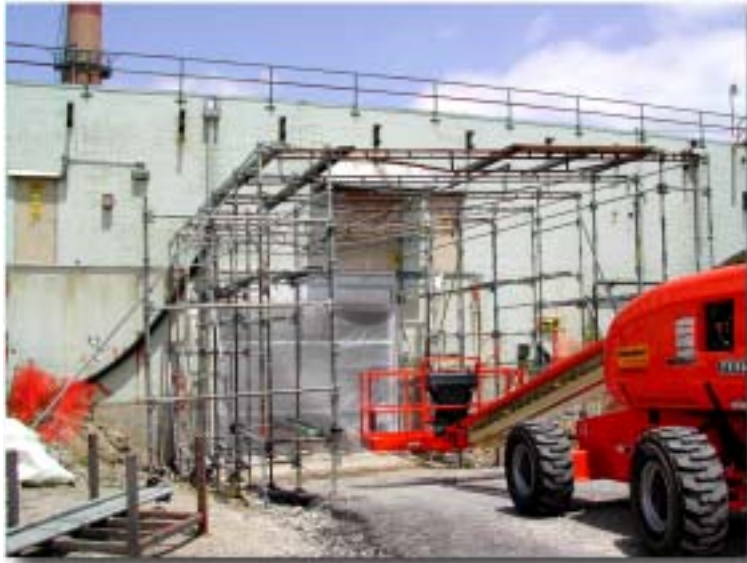
Figure 4-1. The worker fell from the top of this steel-frame scaffold
