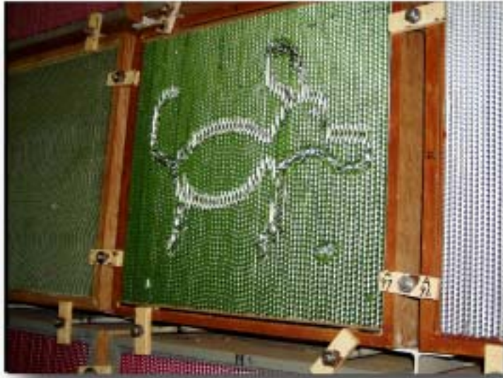
Figure 3-1. One of the defaced HEPA filters
