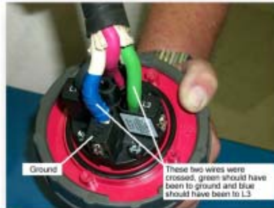
Figure 1-3. Wiring error caused shock
