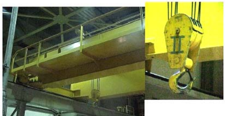
Figure 2-1. 25-ton bridge crane
