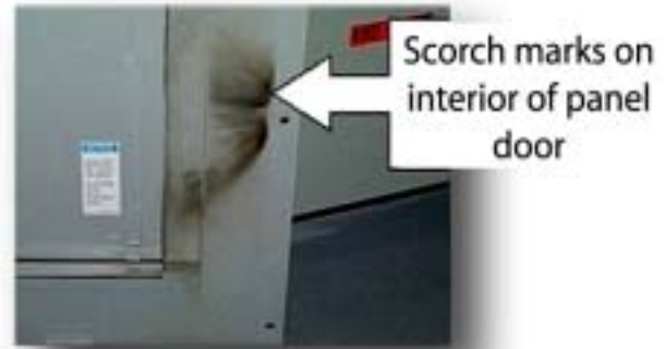
Figure 1-2. The panel door after the arc flash
