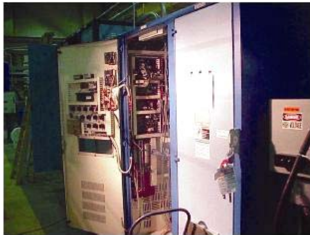
Figure 2-2. Damaged equipment cabinet
