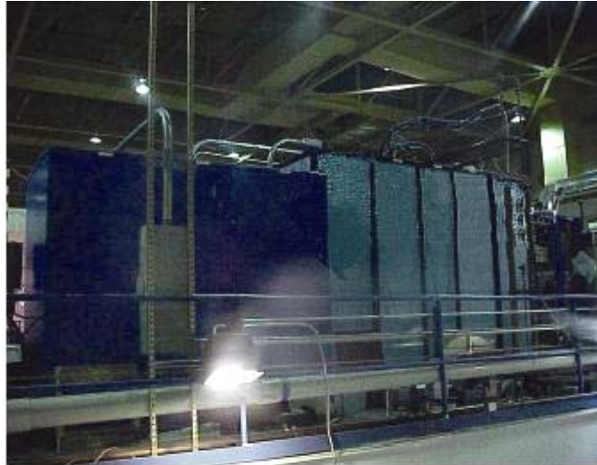
Front and rear sides of damaged cabinet
