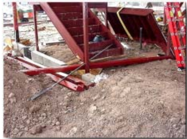
Figure 2-2. Construction site ground level after accident
