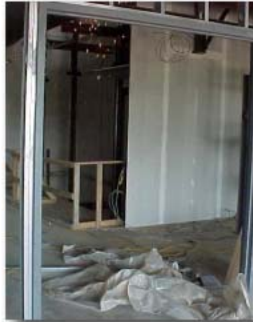
Figure 4-2. Sparks falling onto combustible material
