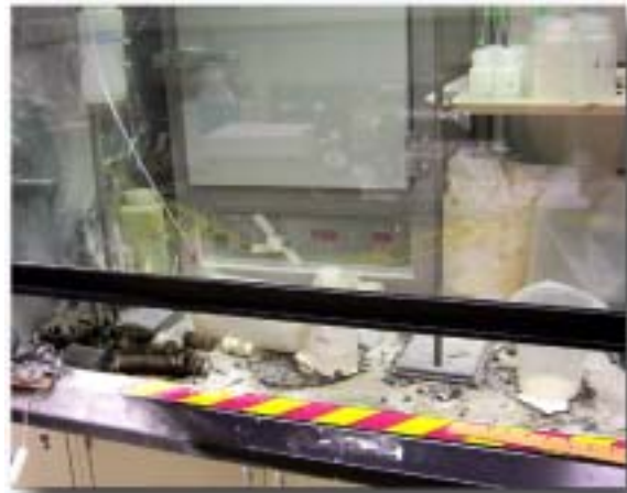
Figure 1-1. Fire damage within the fume hood
