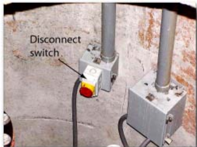
Figure 2-1. Disconnect switch for motor-operated valve
