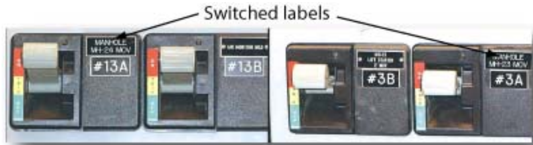
Figure 2-2. Corrected labels for breakers #13A and #3A
