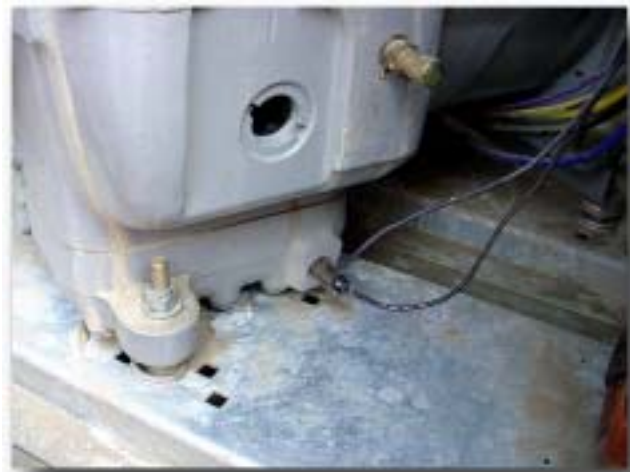
Figure 4-1. Wiring that was shorted to ground
