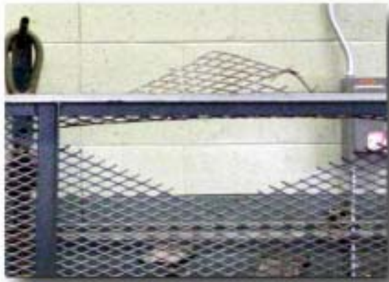
Figure 3-1. The torn protective cage
