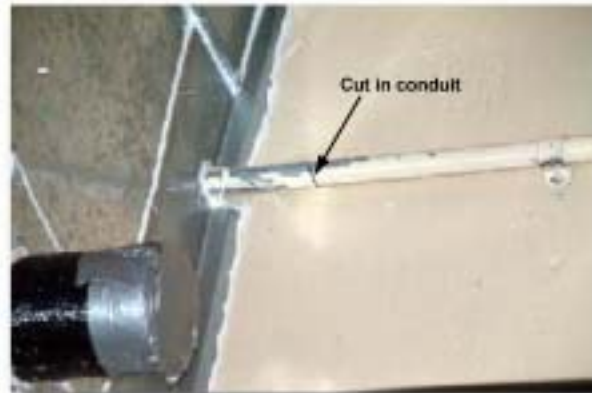
Figure 5-1. Partially cut conduit
