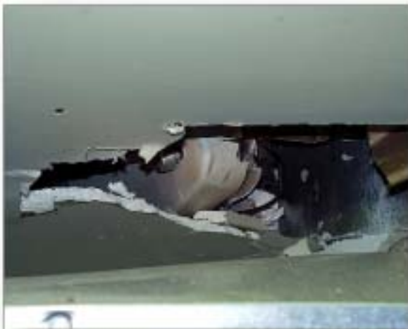
Figure 1-3. The shroud over the Parr vessel protruding from the ceiling
