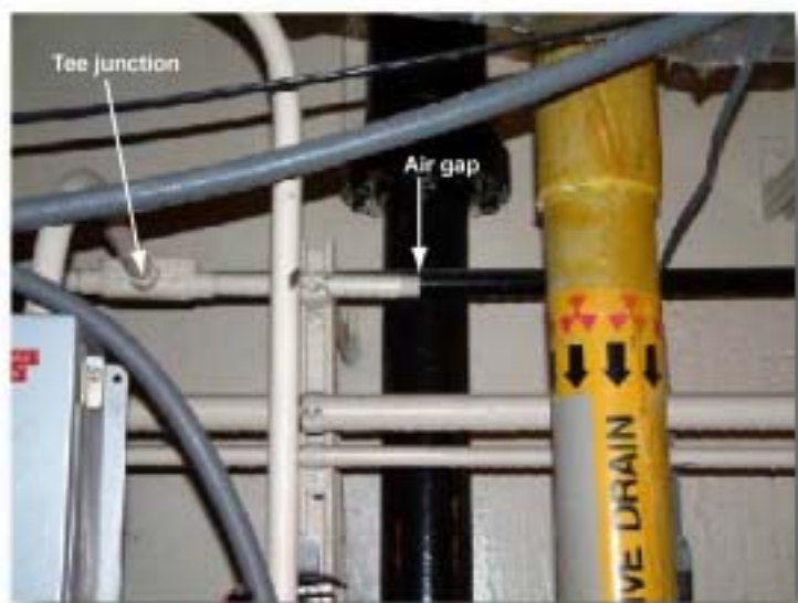
Figure 5-2. Air gap in conduit and tee junction
