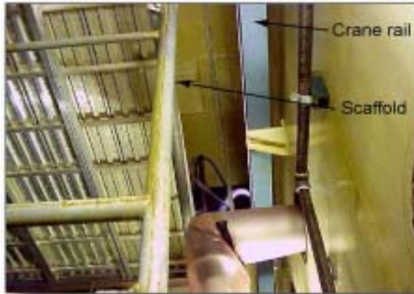
Figure 3-2. Gap between the scaffold and the crane rail
