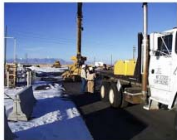
Figure 2-2. Truck with a secured counterweight
