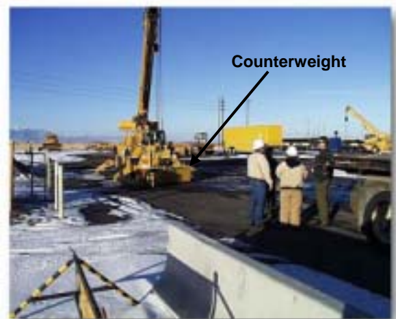
Figure 2-1. Crane and fallen counterweight
