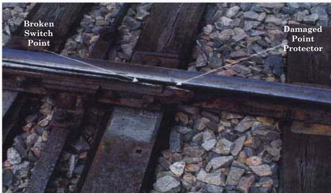
Figure 1-1. Broken Switch Point and Point Protector
