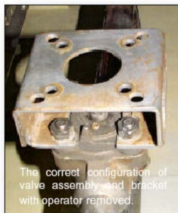
Figure 1-2. Bracket attached to the valve bonnet with the actuator removed
