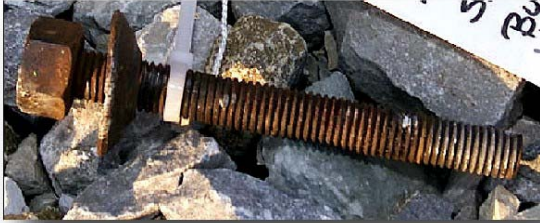
Figure 3-3. Hold-down stud with damaged threads on the right
