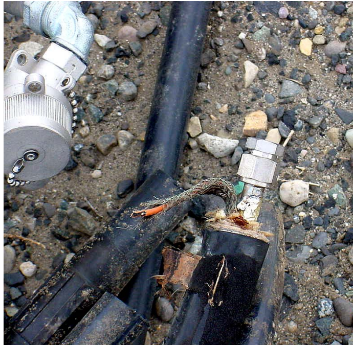
Figure 1. The cut heat trace wires
