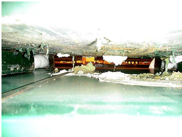
Figure 1. Material leaking from container
