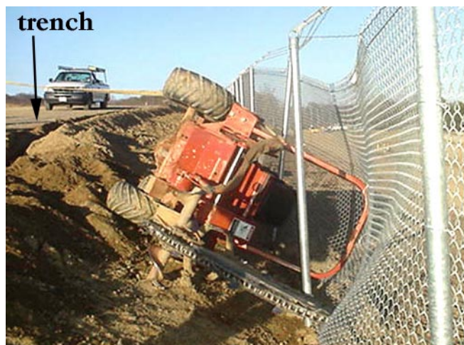
Figure 1. The trencher slid down the slope and was caught by the fence
