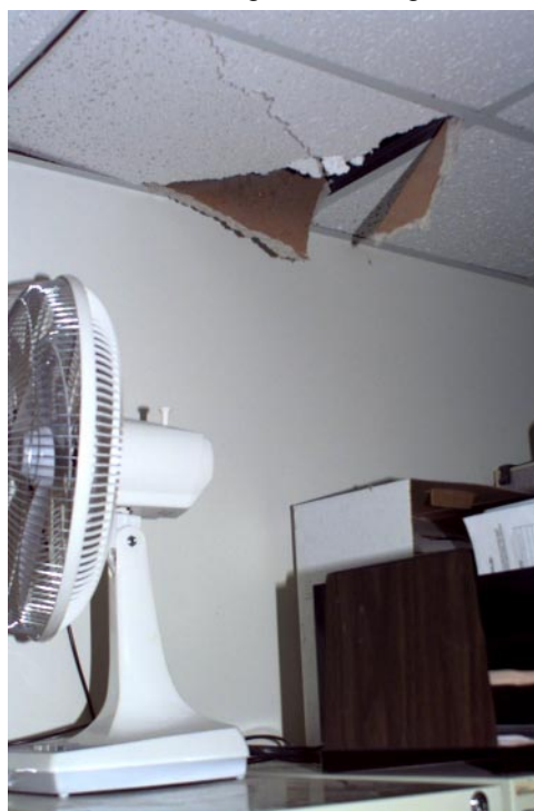
Figure 2. Damaged ceiling tile and filing cabinet where plug came to rest
