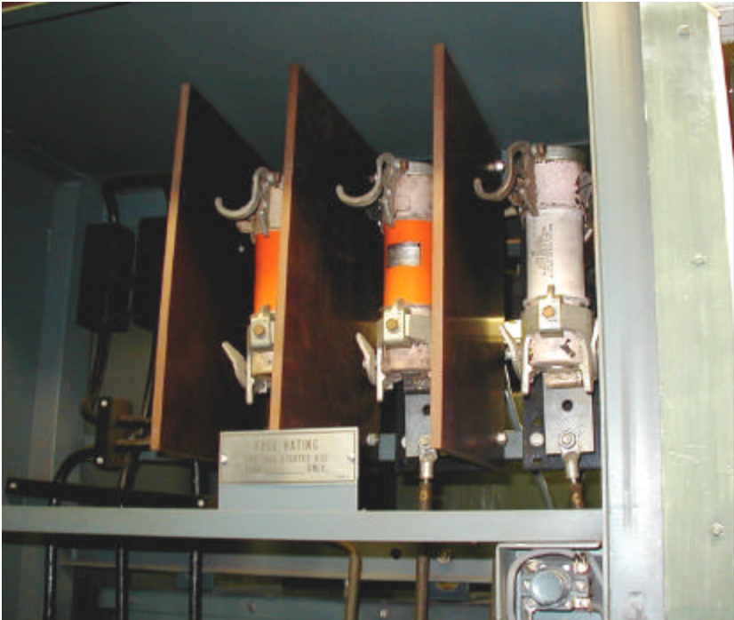
Figure 1. Westinghouse switchgear cabinet showing fuses and their recommended rating
