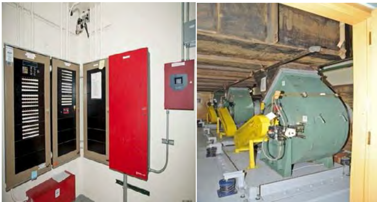
Figure 8: Left: fire alarm control panel installed as part of the TA-55 Reinvestment Project. Right: typical exhaust fan used in the ventilation system.
