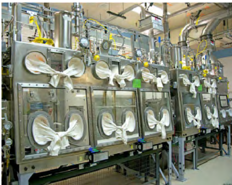
Figure 5. Gloveboxes installed at the Plutonium Facility at Los Alamos National Laboratory.
