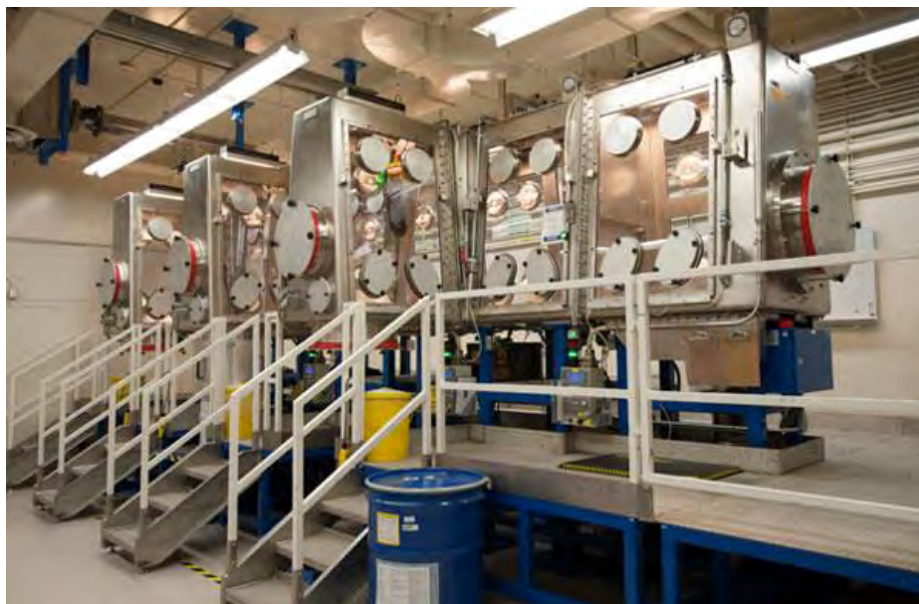
Figure 18. Centralized Waste Processing Line gloveboxes in the Plutonium Facility.
