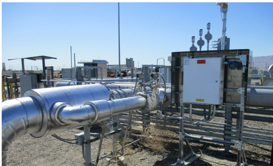
Double-Shell Tank Safety Significant Air Flow Monitoring Equipment
