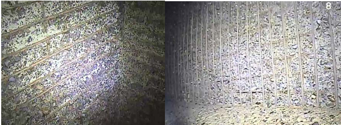
Figure 2. Stills from 2014 crawler inspection video showing two layers of exposed rebar. Degraded concrete debris can be seen accumulated at the bottom of the wall (right).
