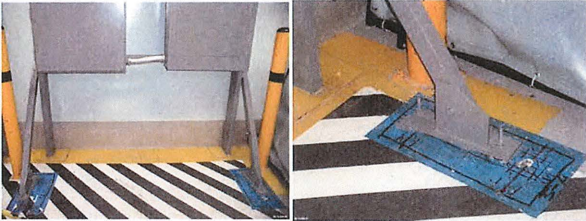
Figure 7. Anchorage of Uninterruptible Power Supply Auto Transfer Switch
