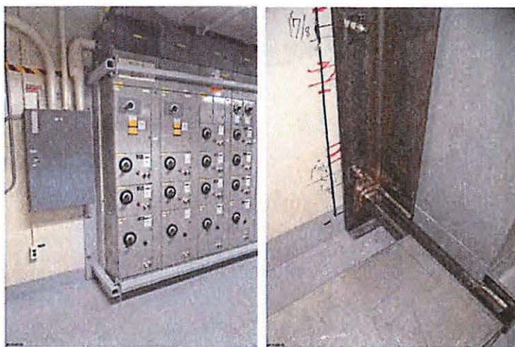
Figure 6. Motor Control System Anchorage
