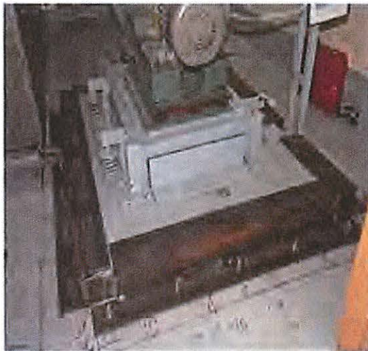
Figure 4. Glovebox Exhaust Fan and Concrete Base Pad with Bracing shown on the Perimeter of the Fan Pad
