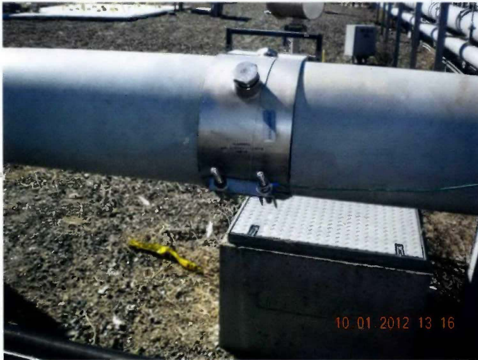
Figure 5: SY Farm Primary Ventilation Duct Flow Test Ports
