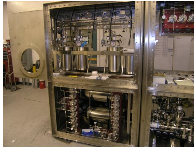
Tritium Processing Station, Lawrence Livermore National Laboratory
