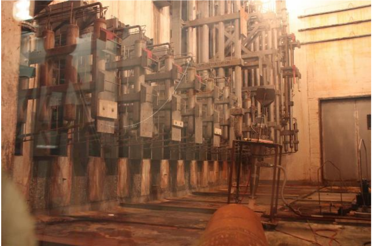
Highly Contaminated Equipment at the Hanford Plutonium Finishing Plant
