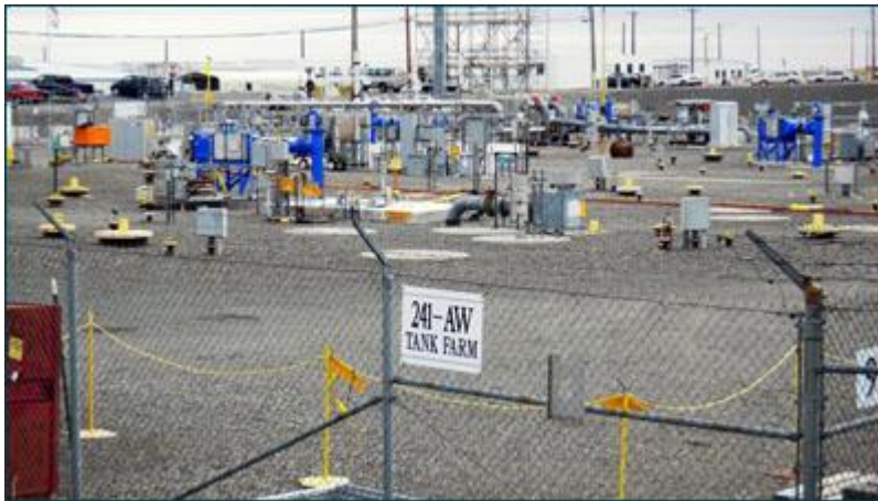
Hanford Double-Shell Tank Farm
