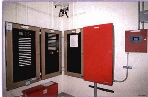
Figure 13. Fire Alarm Control Panels
