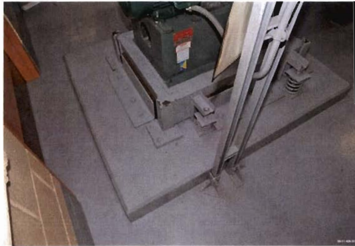
Figure 7. Glovebox Exhaust Fan and Concrete Base Pad
