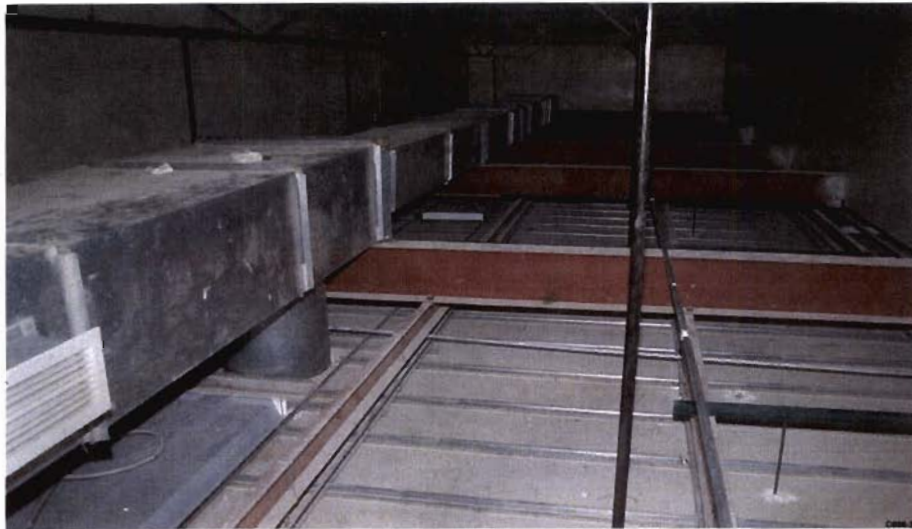
Figure 6. Ceiling Beams (I Beam, top right of photo; C Channel, right center of photo)
