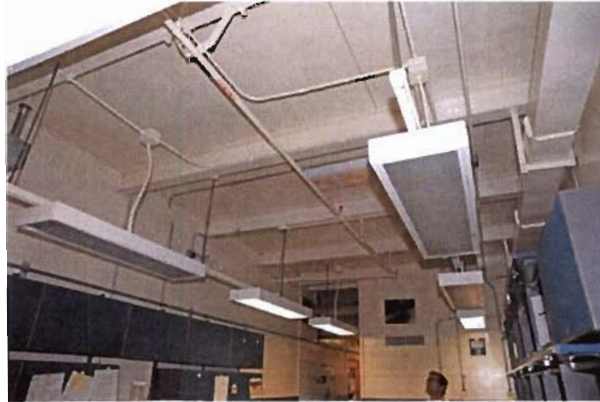
Figure 5. View of Bottom of Mezzanine (Beams to be installed for additional support)
