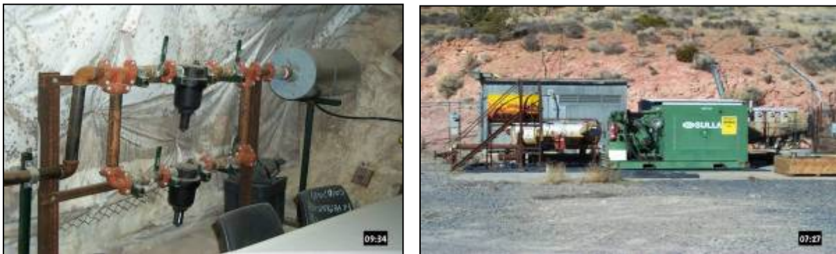
Figure 5-6. Compressed air for U12g Tunnel operations.
