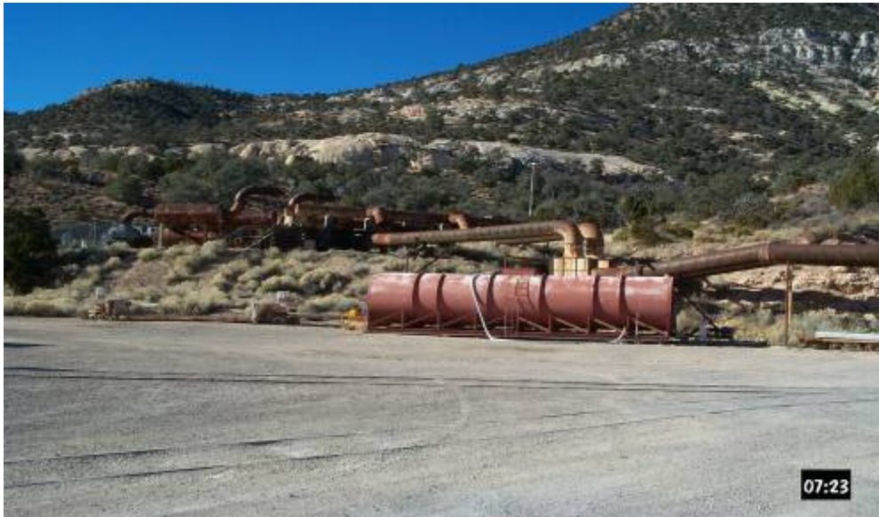
Figure 5-7. U12g Tunnel 16,000-gallon water tank.
