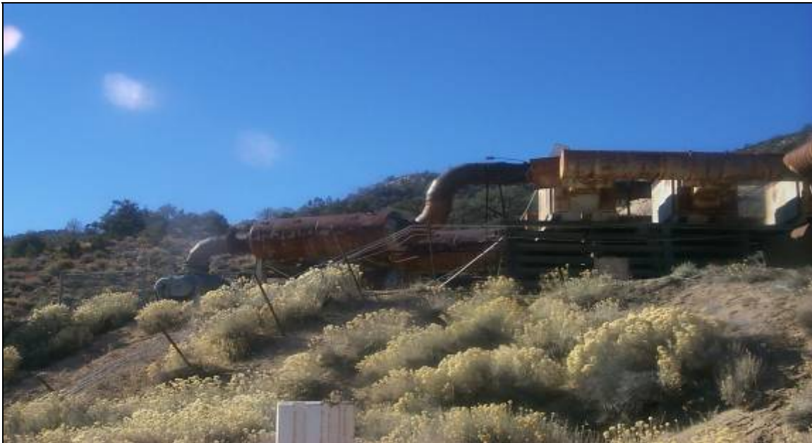
Figure 4-1. Dual 300-hp Sutorbilt Ventilation Fans.
