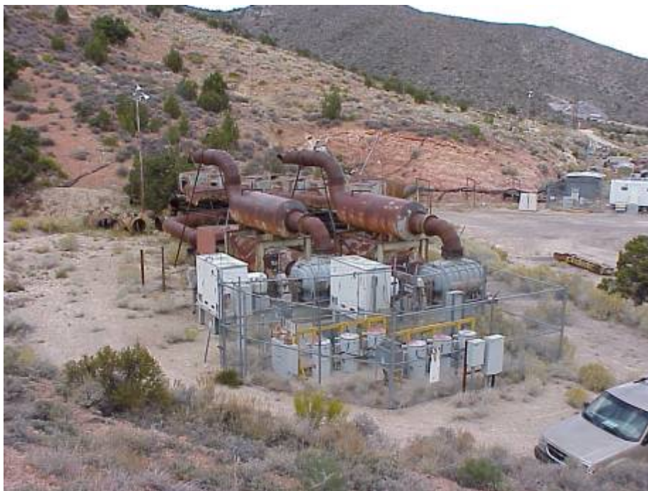
Figure 5-1. Sutorbilt ventilation fans.
