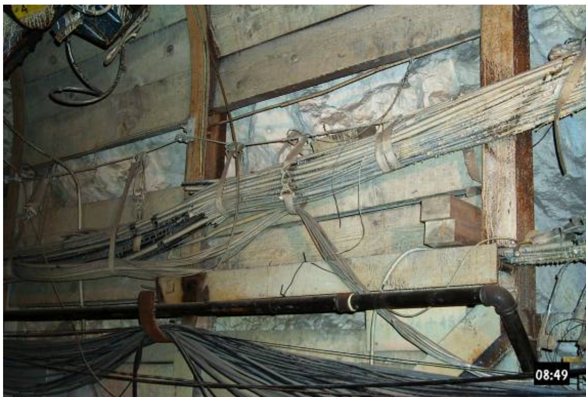
Figure 4-7. Abandoned electrical wiring scheduled for removal.
